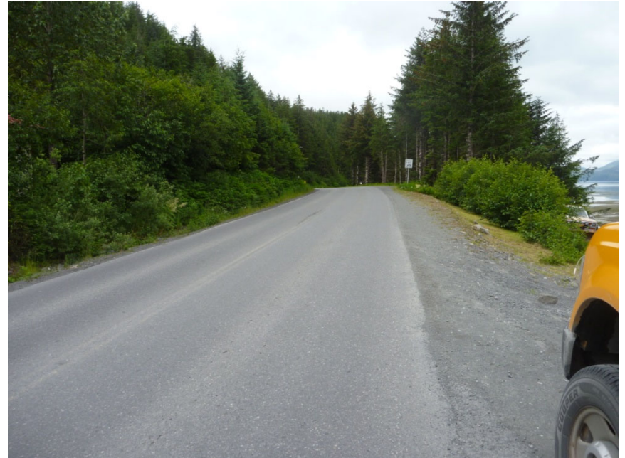
Looking west on Whitshed Road away from Cordova city center. Narrow roadway lanes, no shoulders or pedestrian facilities, steep mountain face on the left, steep drop to the ocean on the right.
