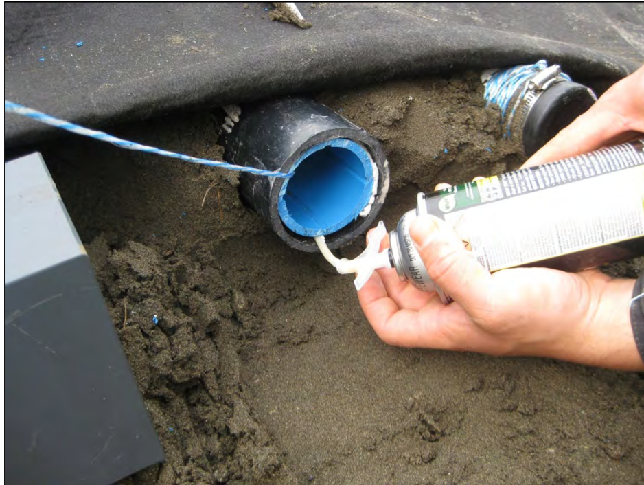
Figure C-16. Filling annulus space with expanding foam to seal outer ABS end cap adapter in place. (Photograph courtesy of J. Zottola, July 2012)
