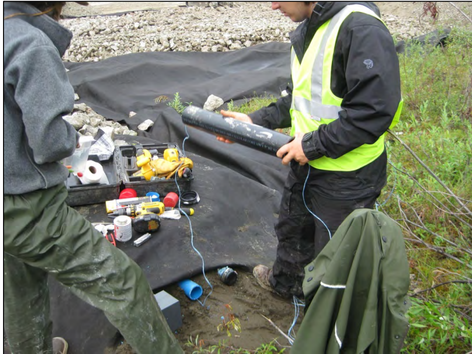
Figure C-14. Routing pull rope for SAA through ABS end cap adapter. (Photograph courtesy of J. Zottola, July 2012)
