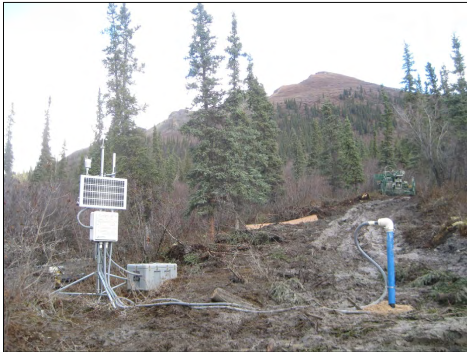
Figure D-7. Completed ADAS location and casing installation of TH12-9004. (Photograph by M. Darrow, Sept. 2012)
