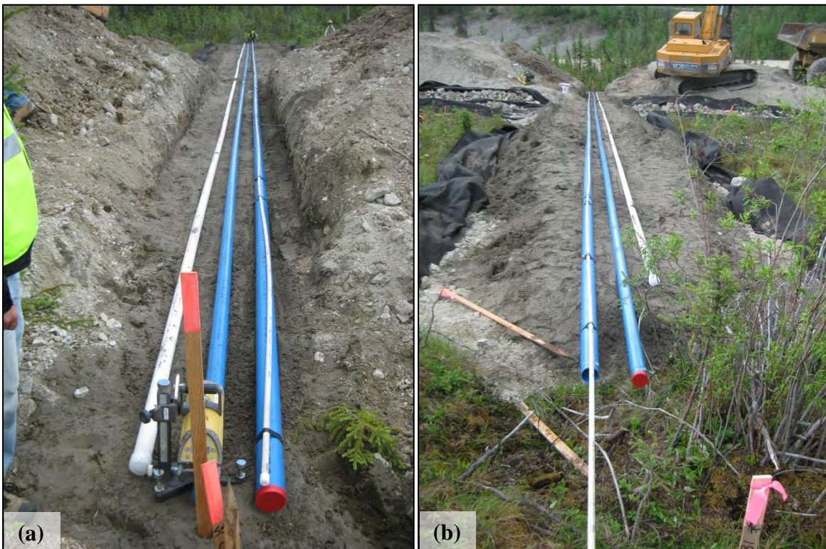
Figure C-2. Casings prior to backfill at the instrumented cross section, looking (a) upslope and (b) downslope. (Photographs by M. Darrow, June 2012)
