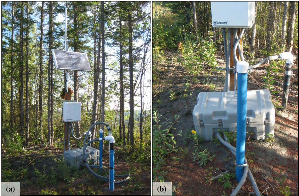
Figure A-19. Final configuration of the Rich113 site. (a) Complete ADAS overview; (b) TH07-1711 in foreground with battery box and ADAS; TH09-1511 is to the right. (Photographs by M. Darrow, Aug. 2011)
