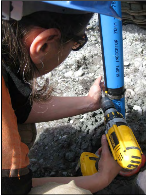
Figure B-3. Attaching the coaxial (TDR) cable with hose clamps at 10-ft intervals. (Photograph courtesy of T. Haller, June 2010)
