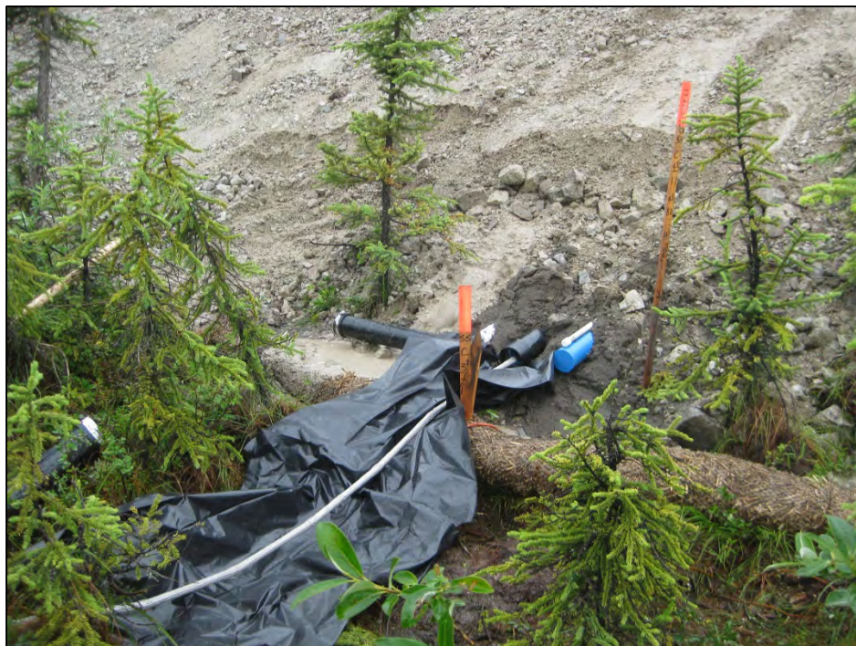
Figure C-10. Installing the SAA device from the downslope end, pulling from the upslope end. (Photograph by M. Darrow, July 2012)
