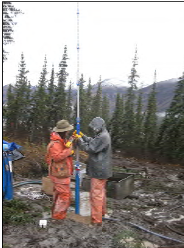
Figure D-4. Installing the INC500 within the guide casing in TH12-9004. (Photograph by J. Simpson, Sept. 2012)
