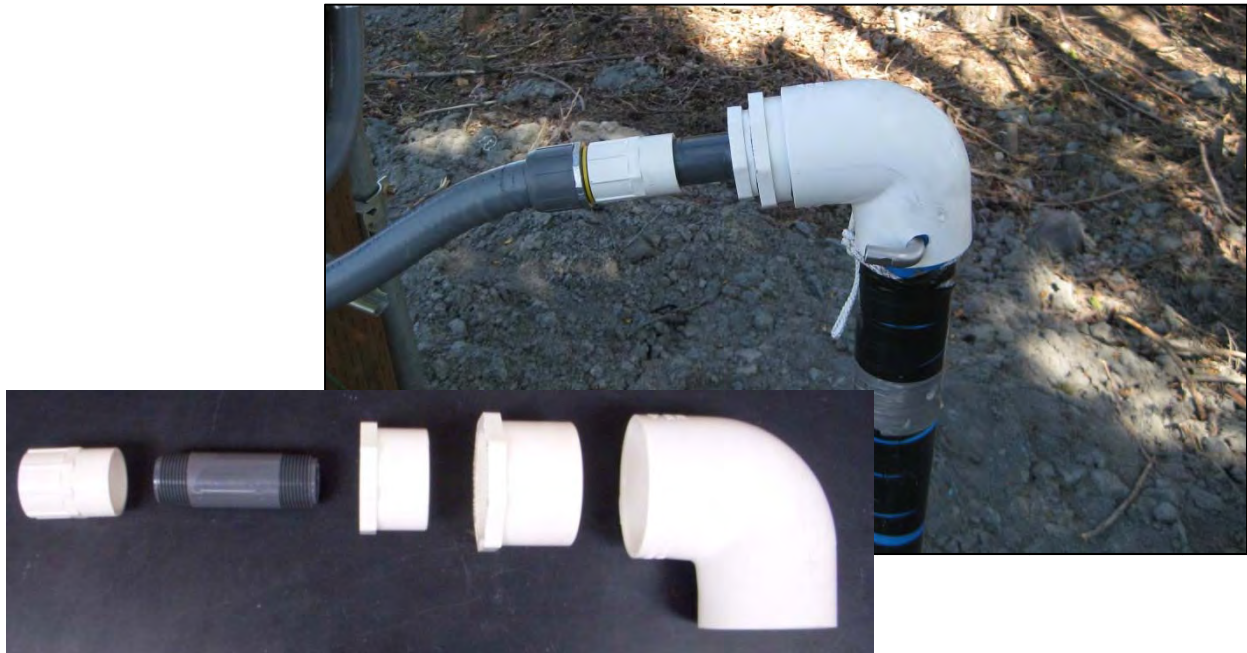
Figure A-18. Guide casing to flexible conduit adapter in place on TH09-1511 casing. Inset illustrates the various PVC fittings that comprise the adapter. (Photographs by M. Darrow, May 2010)
