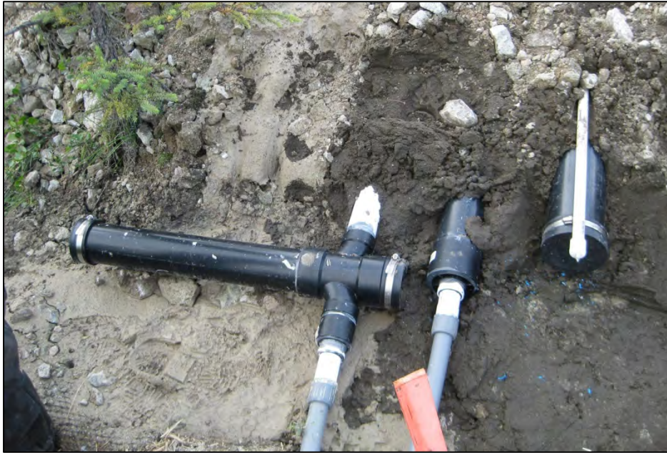
Figure C-24. Downslope casing ends secured. From left to right, ABS casing to flexible conduit adapters for TAC/thermistor cables and SAA device, and sealed guide casing for manual inclinometer probe measurements. (Photograph by M. Darrow, July 2012)
