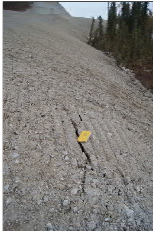
Figure C-27. Cracks in the thermal berm on September 14, 2012. (Photograph by D. Jensen)
