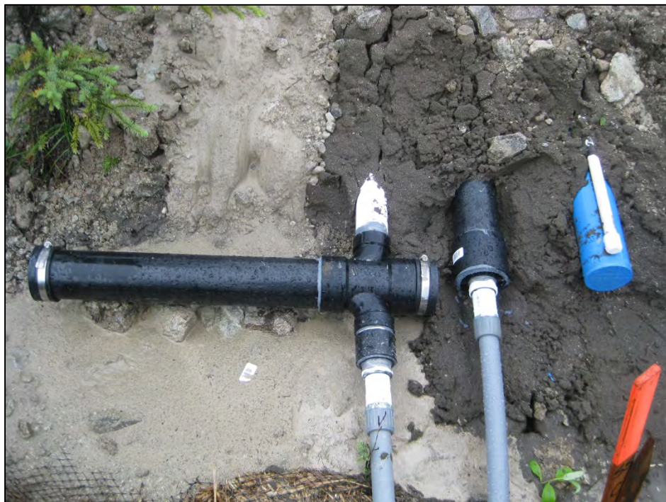
Figure C-12. PVC casing to flexible conduit adapter for SAA installation. (Photograph by M. Darrow, July 2012)
