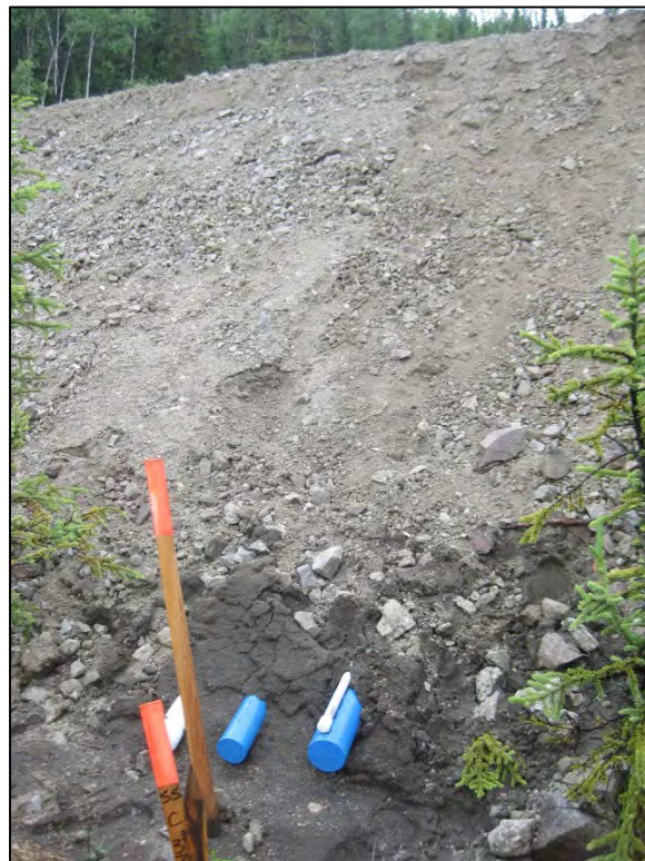
Figure C-4. Downhill toe of embankment with thermal berm and exposed casing ends. (Photograph by M. Darrow, July 2012)
