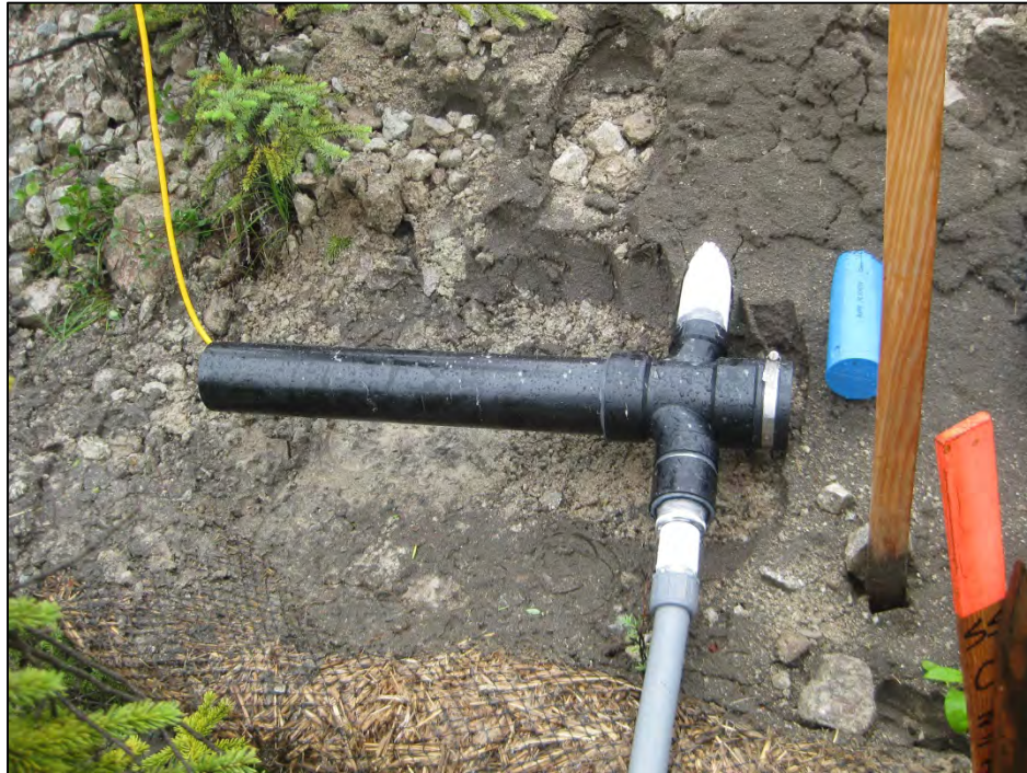
Figure C-9. PVC casing to flexible conduit adapter for the temperature measurement cables. (Photograph by M. Darrow, July 2012)
