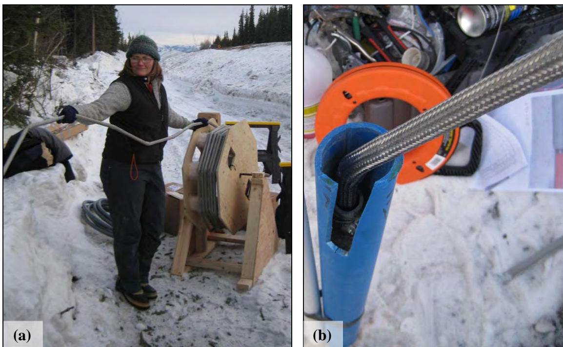
Figure A-15. Installing the SAA device. (a) Guiding the SAA off of the shipment reel, and (b) into the inner 1.05-in. PVC casing. (Photographs by M. Darrow, March 2010)
