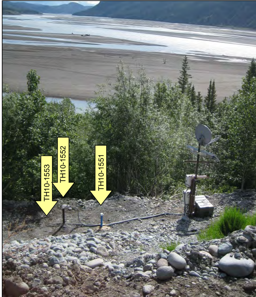
Figure 8. Relative locations of the measured casings and piezometer installation at the Chitina Dump Slide. Vertical arrows are labeled with the test hole identifiers; the installations were located on a drill bench downhill of the roadway embankment. This photograph was taken from the McCarthy Road embankment looking east towards the Copper River. (Photograph by M. Darrow)
