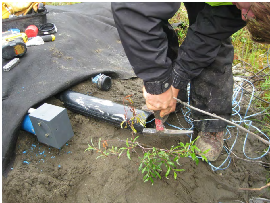
Figure C-15. Tapping ABS end cap adapter into the sand bedding to be flush with inner casing. (Photograph courtesy of J. Zottola, July 2012)
