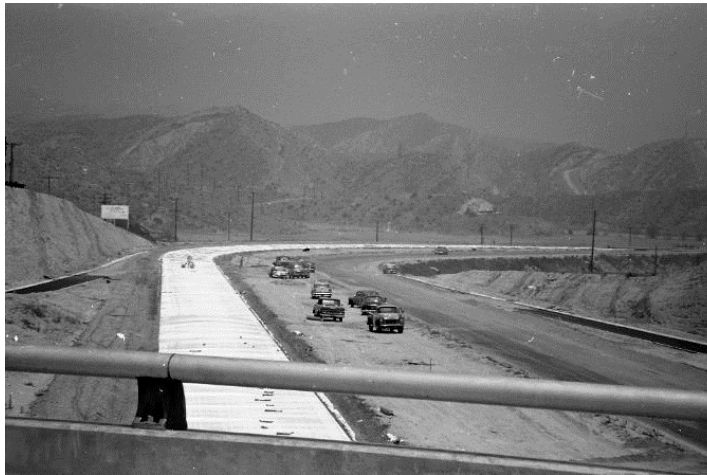
Palmdale, CA – Still in Service
