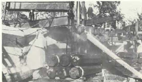
(b) Girder at moment of failure.
