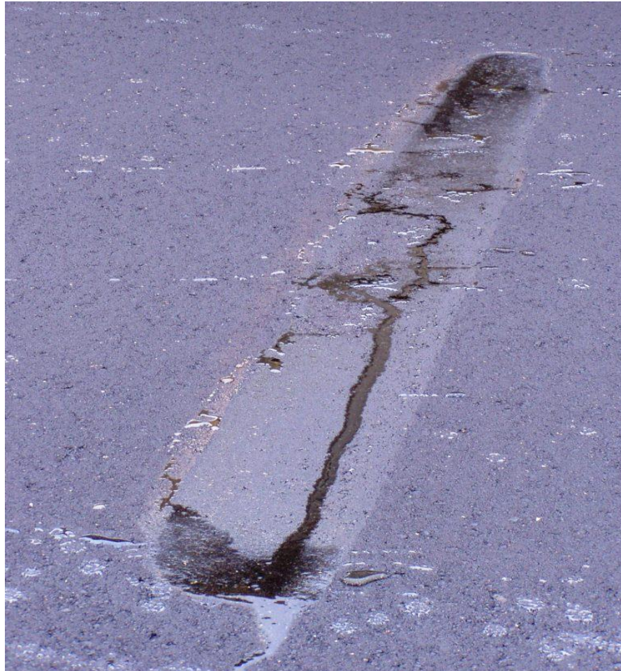
“Birdbath” from roller stopping on hot mat
