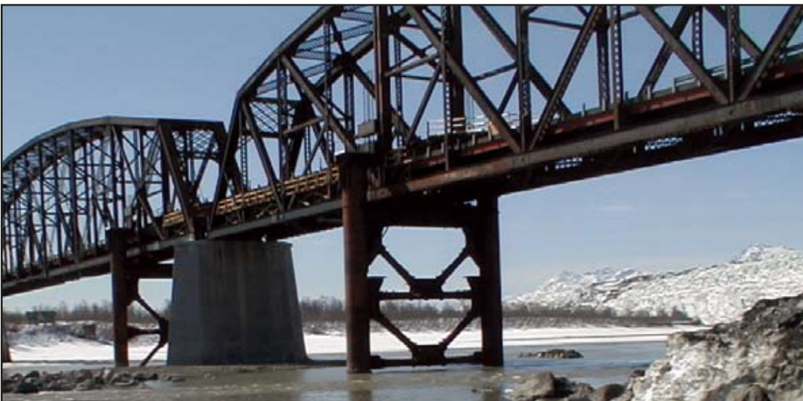
The bridge structure is intact once again with a newly constructed pier. The four pilings used to lift the spans will be removed under phase two of the project.
