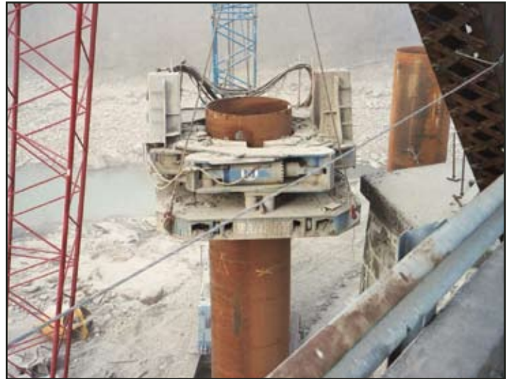
Temporary piling being driven with a hydraulic casing oscillator. Existing material is excavated out of the piling as installed. These piers, four in all, were used to lift both the fallen and intact span, so a replacement pier could be constructed.
