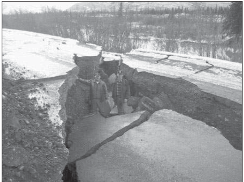
Alaska Dept. of Transportation and Public Facilities Commissioner Joe Perkins inspected the damage that occurred from mile 67 to 78 Tok Cut-off in interior Alaska (see map on page two).
