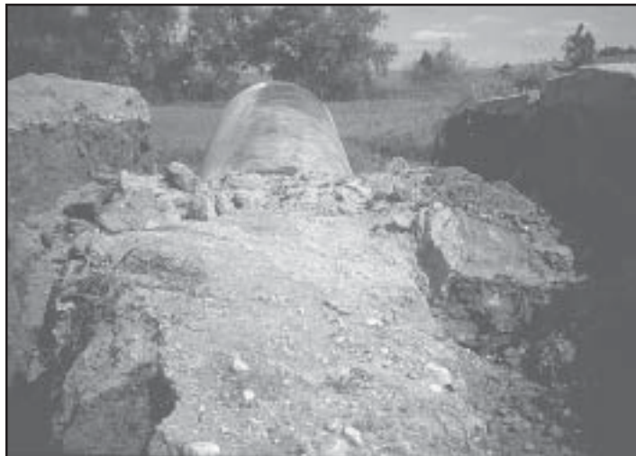
This culvert failed due to installation problems and will have to be replaced.
