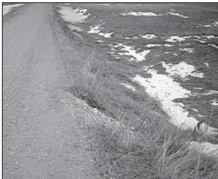
The eroded area at the edge of the road is a hazard and is due to a culvert that is too short and the soil constantly erodes away from the foreslope above it until the road shoulder is affected.
