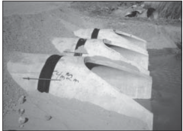
Good example of fabric wrap on the joints of concrete pipe and ties placed between the pipe sections.
