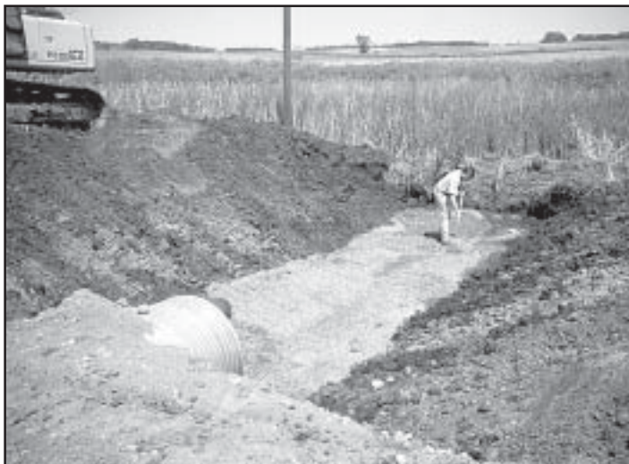
Here is an example of replacing weak and poor soils with good aggregate foundation material prior to setting the new pipe.
