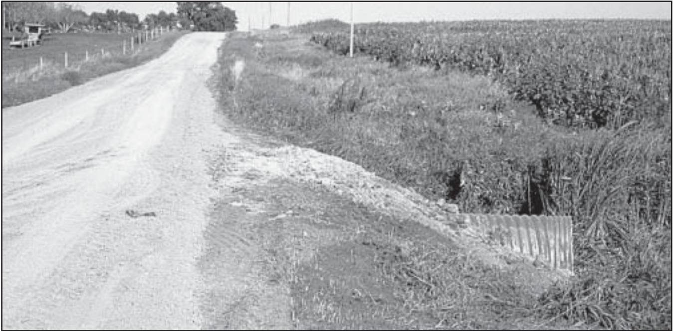
Here is a good example of proper length of culvert so that it extends out to the toe of the foreslope of the roadway.
