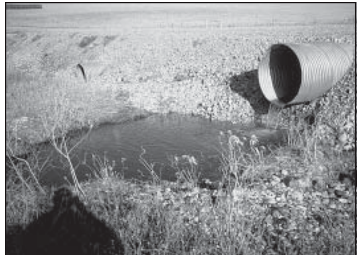
Culvert that was installed without careful check of flow line during installation.
