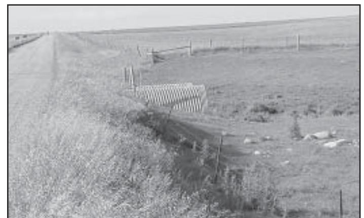
Here is a contrast with a culvert of correct length that extends well out to the toe of the foreslope.
