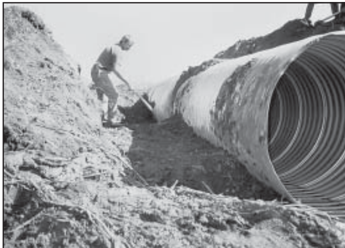
Hand tamping under haunch of pipe is critical to seal the culvert in the backfill soil as well as to prevent deforming of the pipe when loads pass over it after the road is reopened.
