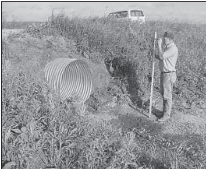
A hand level is used here to determine the height of the grade at the shoulder. This height multiplied by 2 equals a 2:1 foreslope which is the minimum recommendation even on a very low-volume road. The base of the survey rod shows where the end of this pipe should be.
