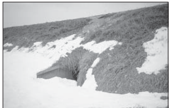
The end of the culvert is nearly hidden at the base of the slope. It is far too short for the height of this grade.
