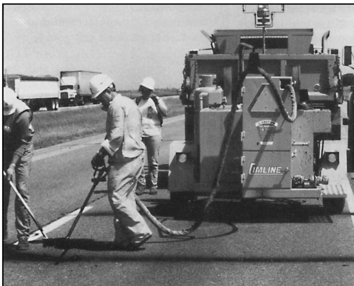
The LTPP program's recently updated Manuals of Practice include information on materials and procedures for pothole repair.
