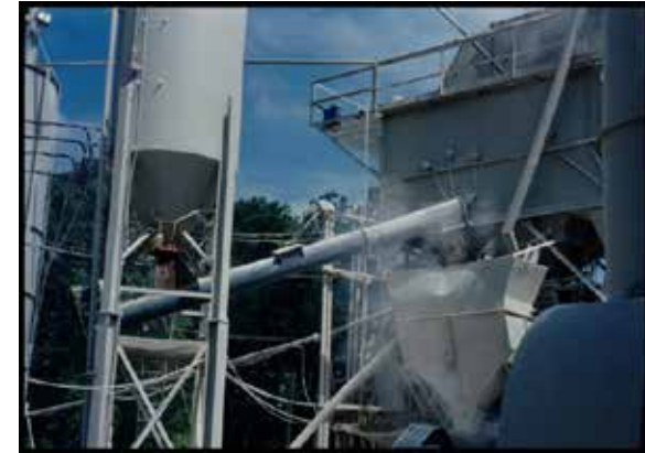
Mineral Filler Silo
