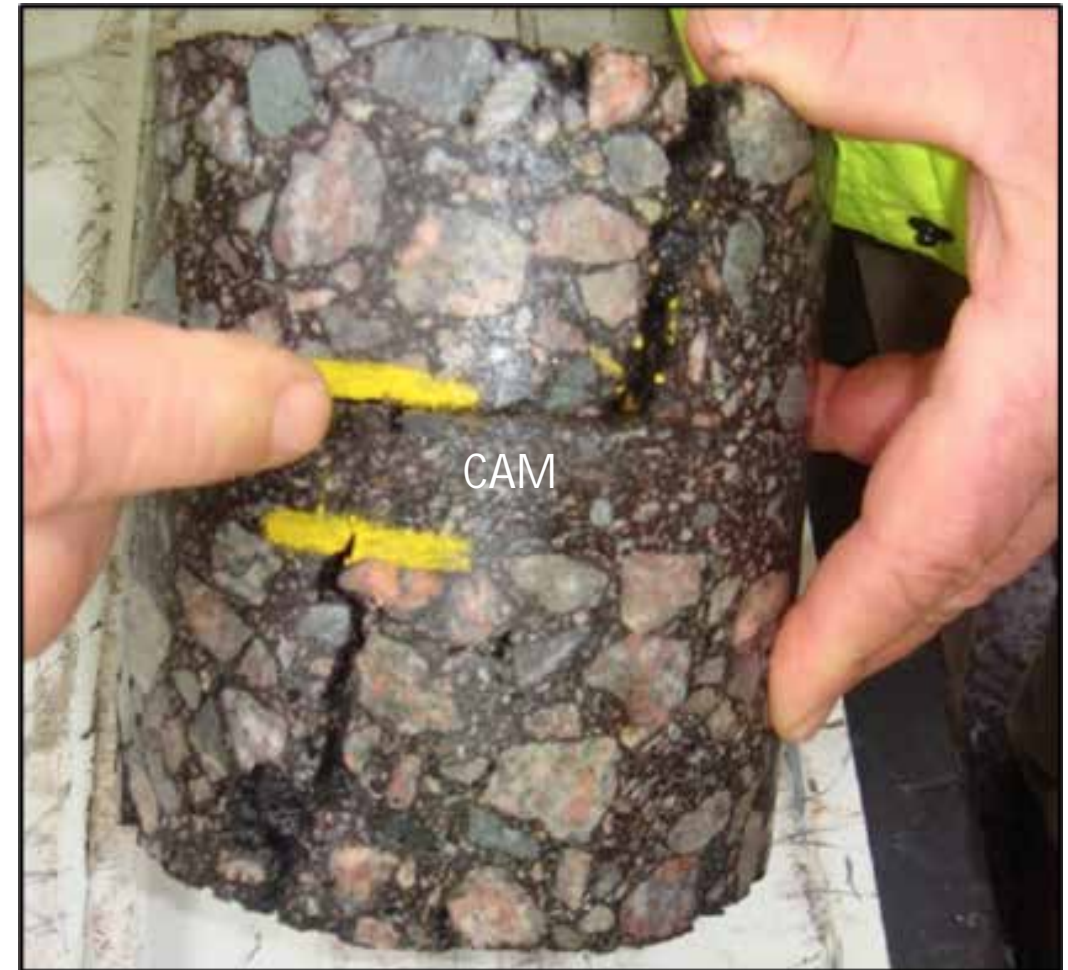
Crack jumping observed in core sample
