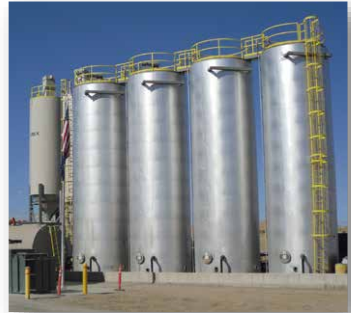
Binder Storage Tanks
