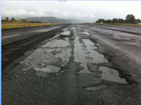
Delamination Between FASBC Layers
