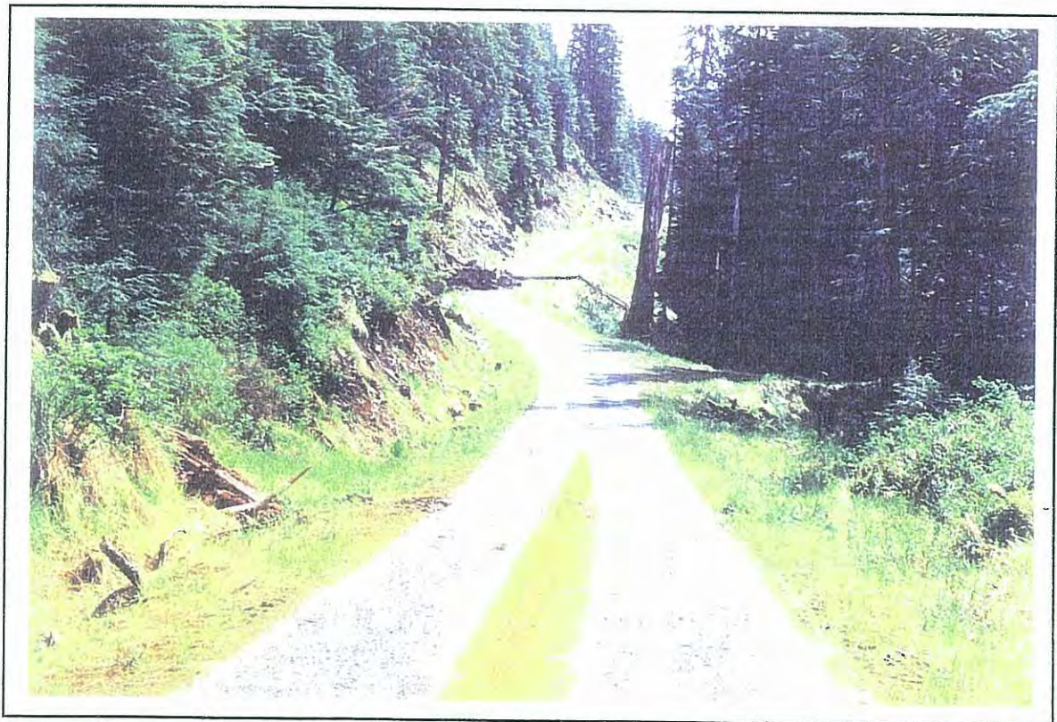
Photo 2 : Typical roadway section showing steep cut slopes in mixed soil and rock common material. Note irregular roadway alignment.
