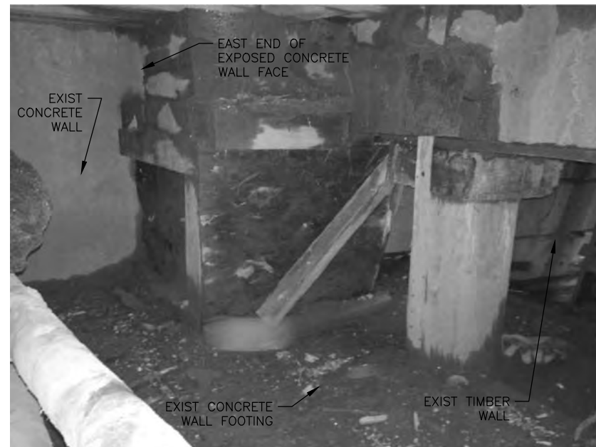
3 PHOTO OF WEST END OF WALL REPLACEMENT LOOKING NE M11 SCALE: NOT TO SCALE
