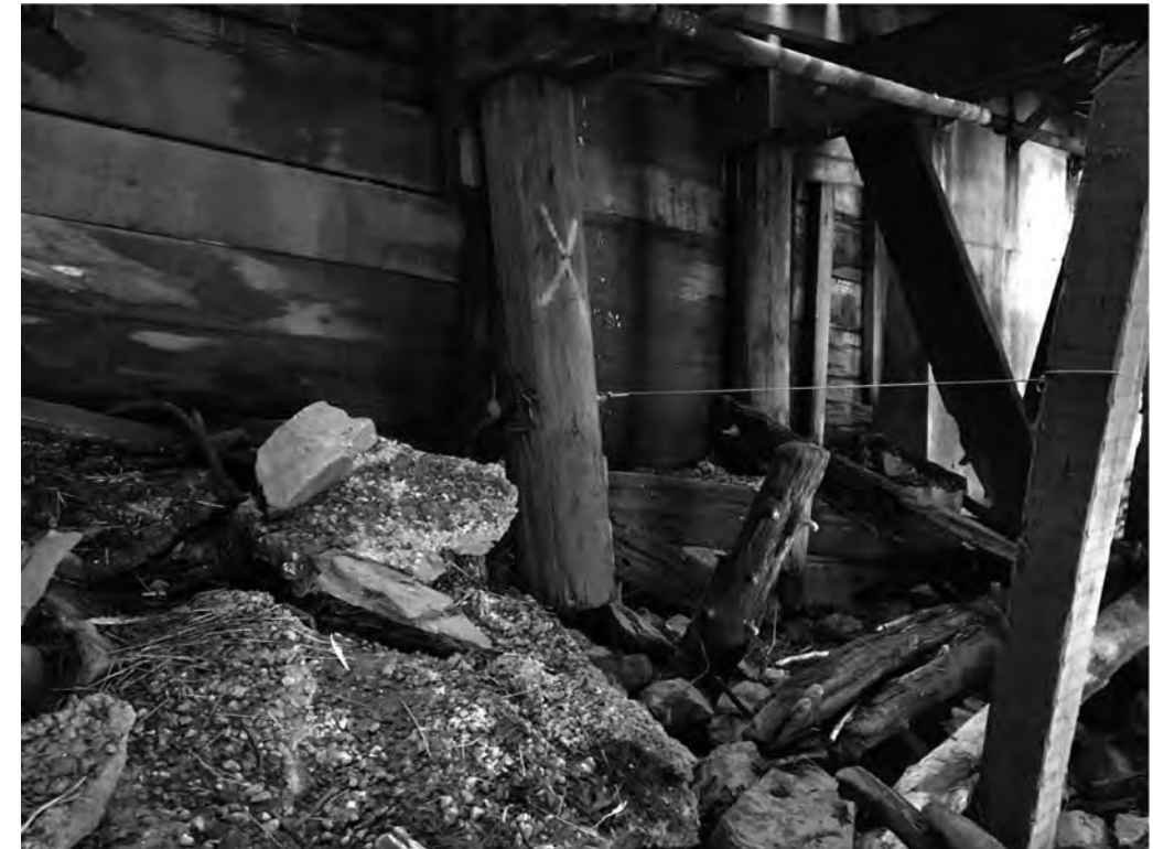
2 PHOTO OF TIMBER WALL (EAST SIDE) LOOKING NE M11 SCALE: NOT TO SCALE
