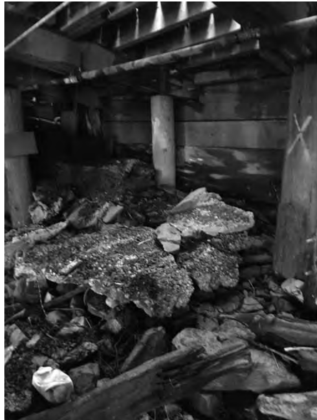
1 PHOTO OF TIMBER WALL (WEST SIDE) M11 SCALE: NOT TO SCALE LOOKING NW
