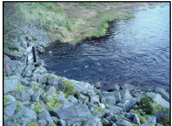
Figure 19 - Auke Nu Creek exiting culvert under Glacier Highway
