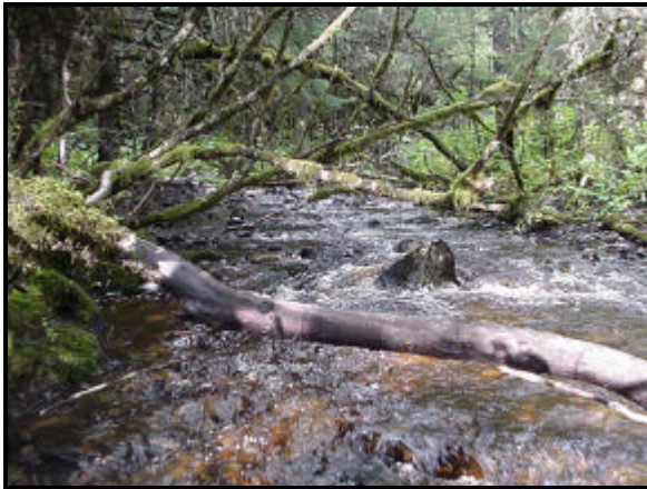
Figure 16 - Auke Nu Creek before entering culvert under Glacier Highway
