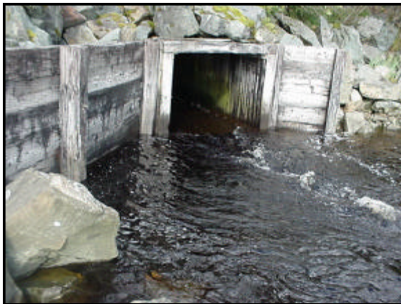
Figure 18 - Auke Nu Creek exiting culvert under Glacier Highway
