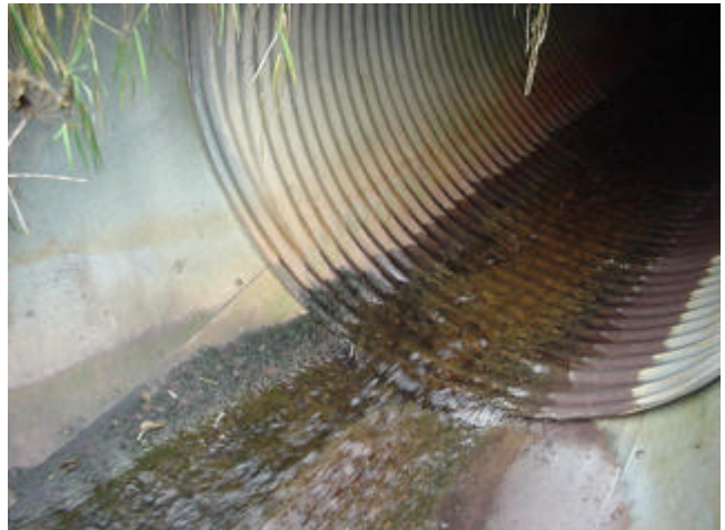
Figure 11 - Bay Creek culvert with algae growth on bottom of pipe
