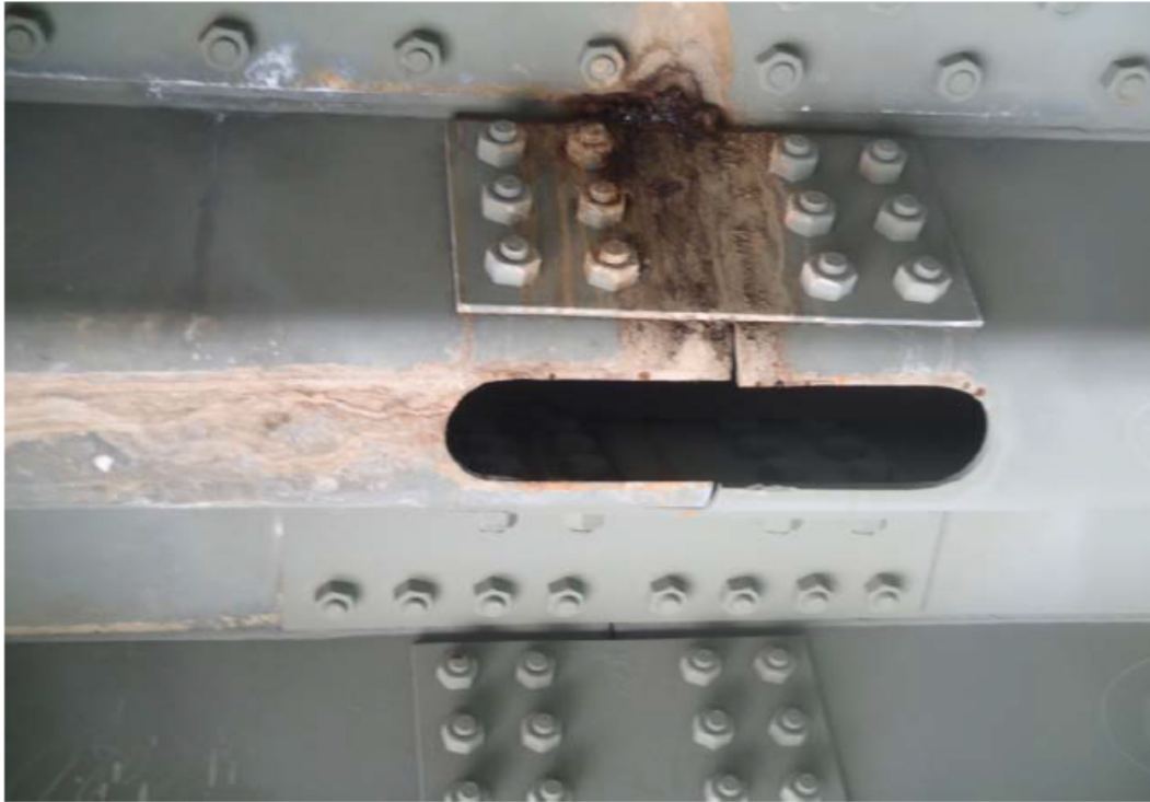
Figure 5-1. Debris on Top Flange and Stiffeners on the Yukon River Bridge
