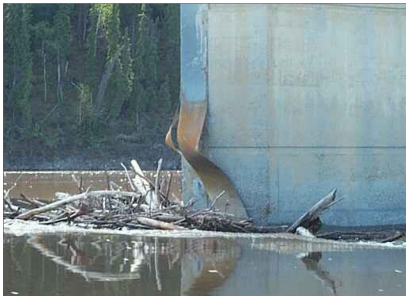
Figure 6-9. Ice Damage to the Yukon River Bridge Steel Pier Nosing
