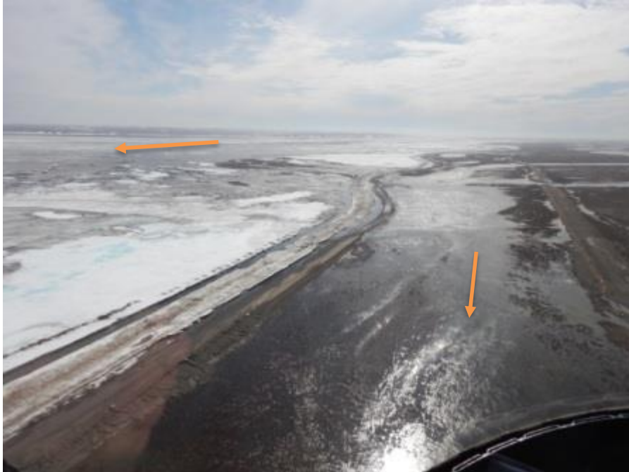
Figure B.9. Photo taken May 27, 2015, near Dalton Highway MP400, view south. Water levels have dropped appreciably, and tundra west of the pipeline (far right) is no longer flooded. Road damage is easily discernable in this photo. A Sagavanirktok River channel is at far left, and Franklin Bluffs are seen on the horizon, upper center.
