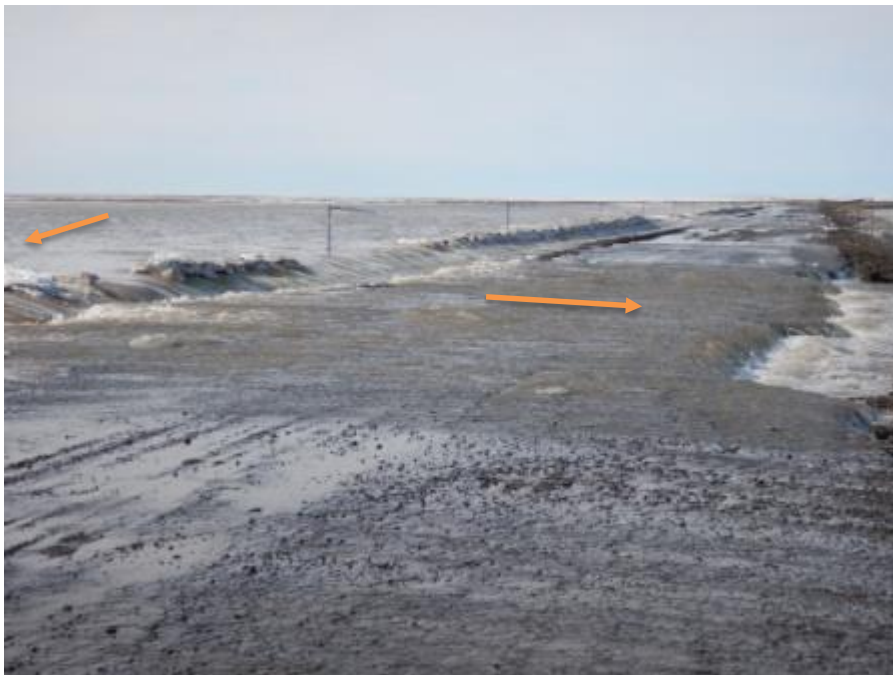
Figure B.14. Photo taken May 17, 2015, near Dalton Highway MP395. View is south and photo shows water at left flowing over afeis accumulation 1–2 ft higher than the road surface. Water continues across road and begins erosion of the west (right) shoulder. Road material is still frozen at this time. This location is the southernmost occurrence of flooding across the road.
