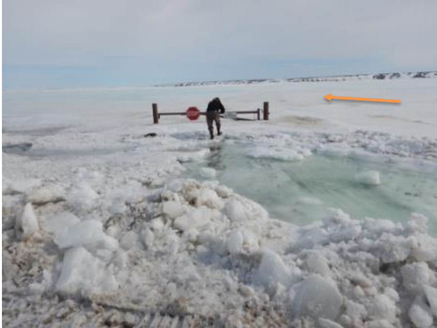
Figure B.11. Photo taken May 15, 2015 at Dalton Highway MP395.5. View is northeast and shows the extensive buildup of aufeis—several feet thick at this location—evidenced by the partially buried Alyeska access gate. Franklin Bluffs can be seen in the background.
