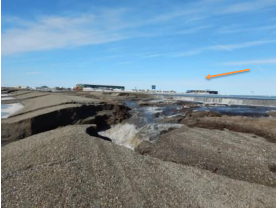
Figure B.1. Photo taken May 19, 2015, near Dalton Highway MP414. View is south and shows accumulated floodwater west of the Dalton over-topping the road surface at right, flowing across tundra in mid-ground, and cutting through a protective gravel berm as the water returns to an active channel of the Sagavanirktok River at the far left of photo.
